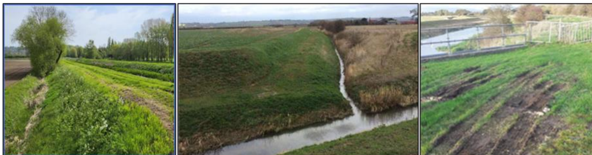
Photo 7: Rutting on crest bank on Carholme Drain; Photo 8: Skinnard Dyke bank reprofiling; Photo 9: location for improved vehicle access at Lincoln Washlands
